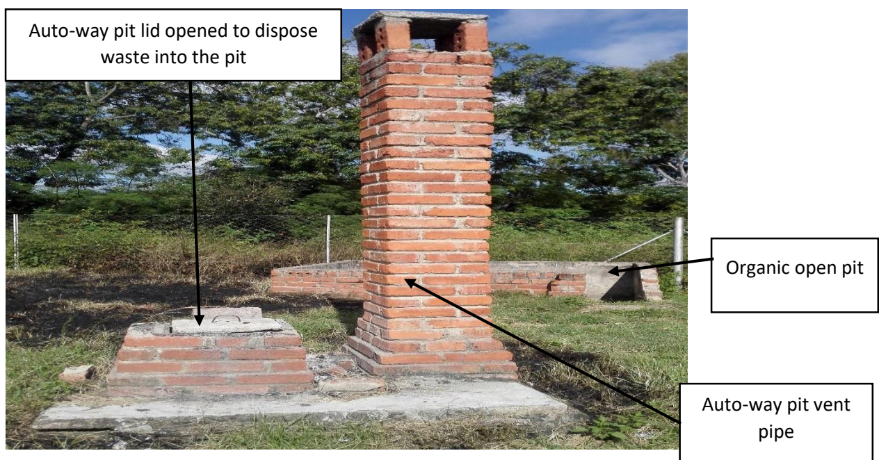
Plate 2: Auto-way pit and organic open pit used to dispose pathological waste and organic waste respectively at STT hospital.
