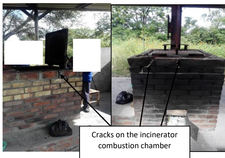
Fig. 28: Cracked incinerator used to dispose solid waste at ST Theresa hospital.
