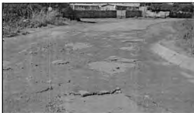
Fig. 4 State of the road at Ziyambi Drive and Matongo Way intersection in Senka-Nehosho area.
