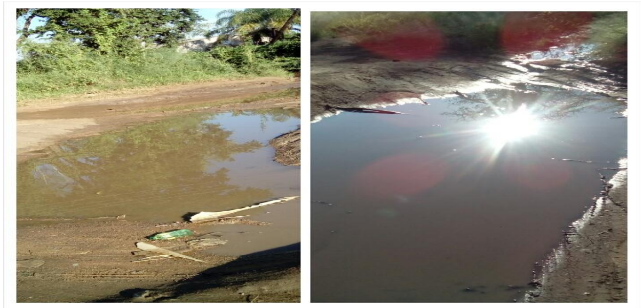
Plate 10 ( Sewer water flooding the gravel roads) Plate 11 (burst water pipe in Tshovani)
