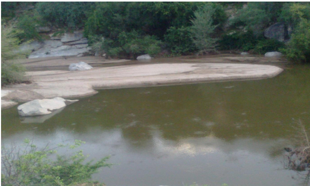
Fig 6: Heavily Silted Changazi Weir Dam
