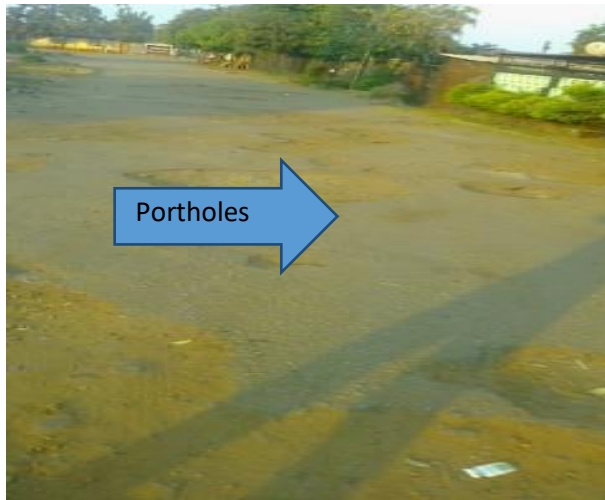
Figure 6 , crumbling roads in Harare, in Highfield high density suburb, 2015
